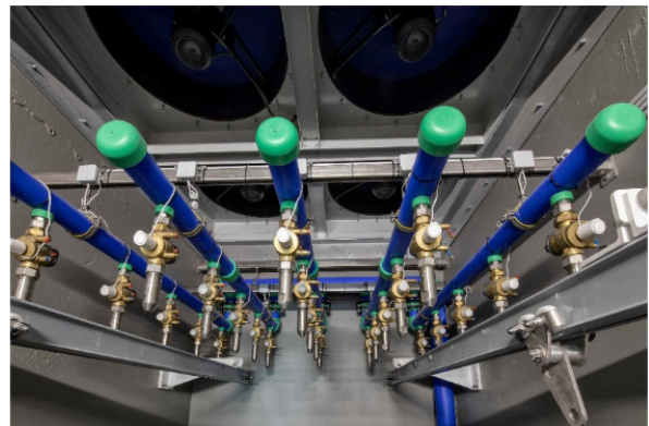
Figure 11 Gravity-activated waterfall system in the Climate Cascade. Photography: Eric Fecken
