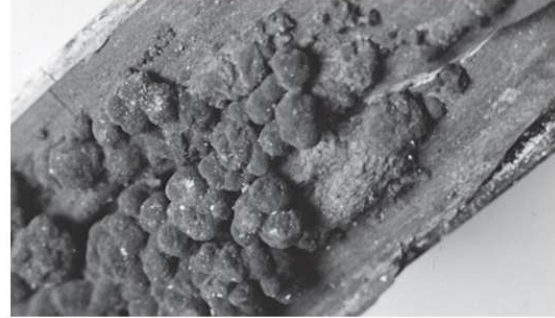
Figure 3.23 If the roof deck is damp for a long time, this can produce entire fungus cultures
