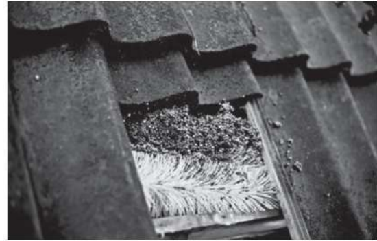
Figure 3.20 When insulating tiled roofs retrospectively, urea formaldehyde foam or compound polystyrene foam flakes are also used. A row of tiles is removed locally and the material is inserted under the tiles with a long lance.
