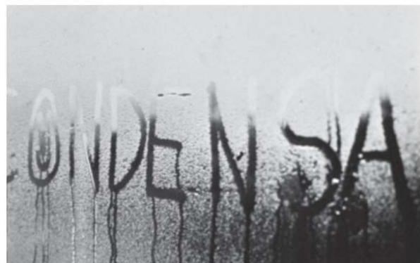
Figure 2.7 If the temperature of the window is lower than the dew point temperature of the air on the inside, then condensation will occur.
