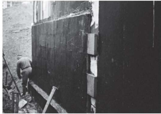
Figure 3.14 Insulation of a cellar wall with foam glass attached with a preparation of bitumen, and finished with bitumen and glass fleece
