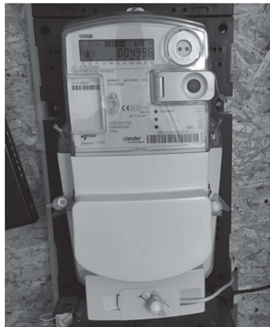
Figure 8.1 Energy meter in a home. Both the gas and electricity use can be read at distance.
