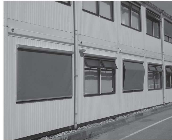
Figure 7.10 The ventilation through open windows or ventilation grids can be seriously hindered by external sunscreens
