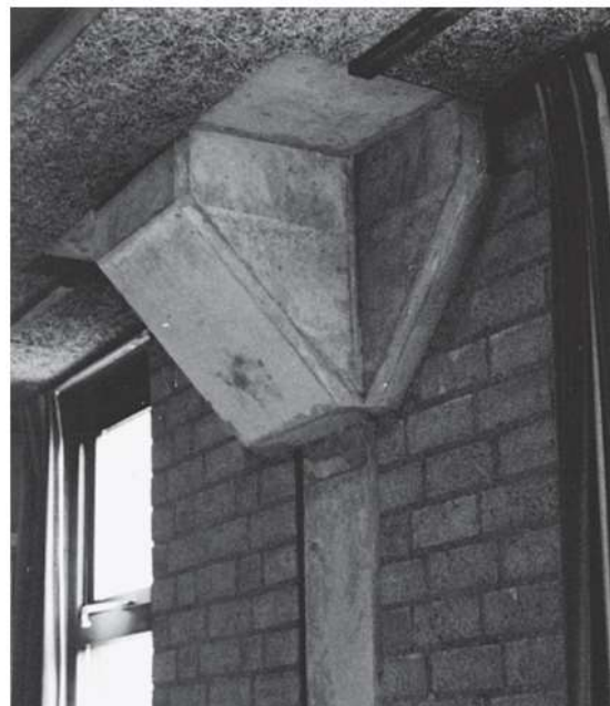
Figure 1.31 The same situation as in figure 1.30, but seen here from the inside
