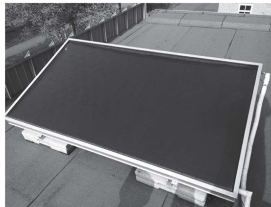
Figure 8.4 A solar boiler on the roof of a home sustainably generates warm tap water (partly)
