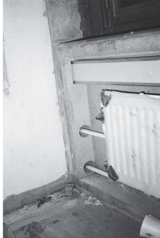
Figure 12.23 Pipe feed-throughs can often cause sound leaks. In this case the feed-throughs have been sealed using (injectable) plastic foam.
