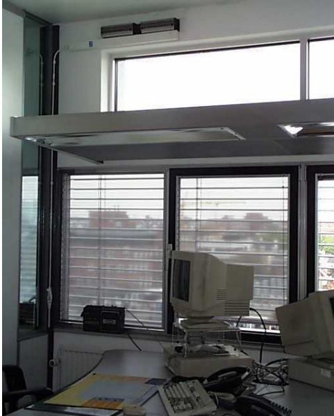
figure 2. the “daylight shelf” (Du.: “lichtplank”) reflects the light against the ceiling, so that it can reach the back of the room; the lower part of the window has sunblinds. In this way the distribution of light in the room is more steady
