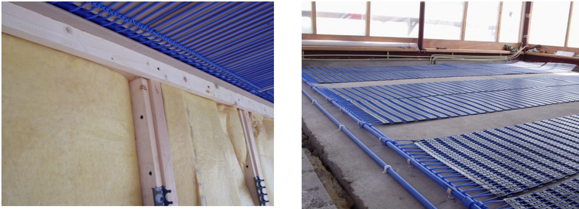
Figure 9: Tubing for concrete surface activation in the ceiling on the left and in the floor on the right.
