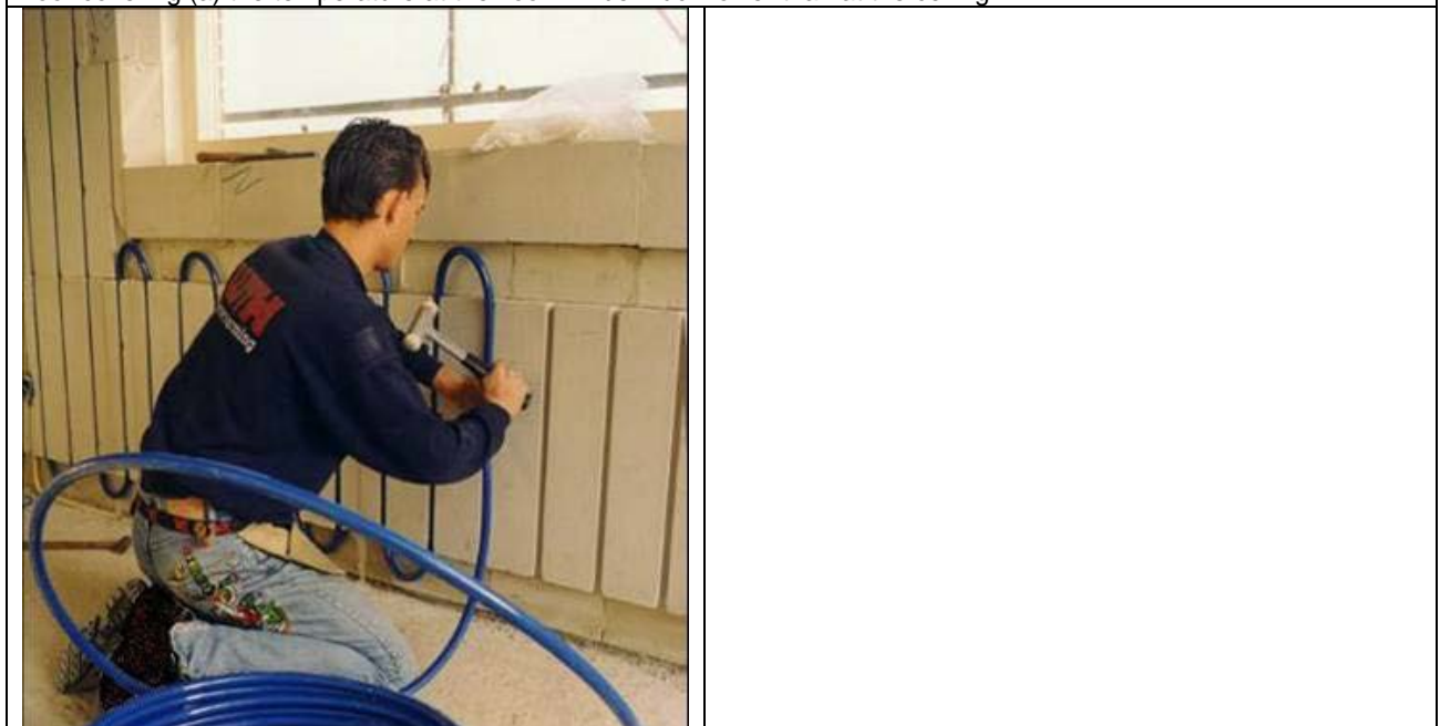
Figure 5: It is possible as well to integrate pipes in a wall. When the wall is a façade, the other side will be insulated and most of the thermal energy will flow to the room.
