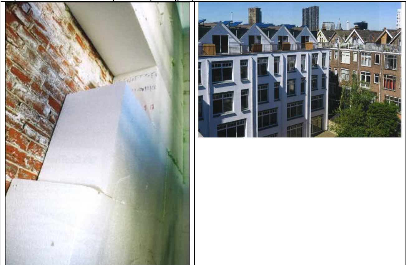
figure 4. example of the application of 30 cm isolation for the renovation of existing houses; the R_c -value of the façade is 10,0 \text{ m}^2\text{K/W} .
